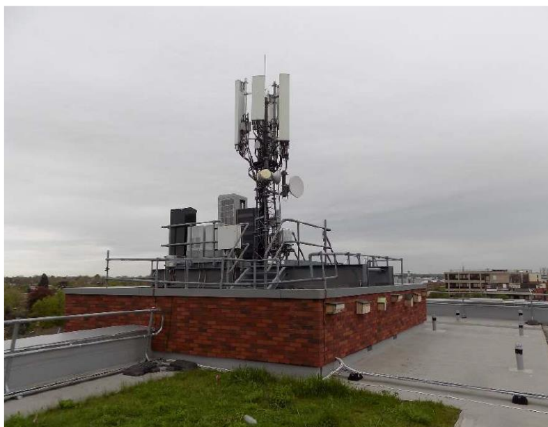
Existing rooftop mast, antennas and cabinets
